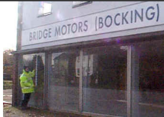
Evidence of flood level on the window of a local garage
