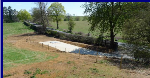
Pinfold Production borehole in operation
