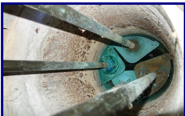
Old Evershed Noflote electrodes monitoring water level
