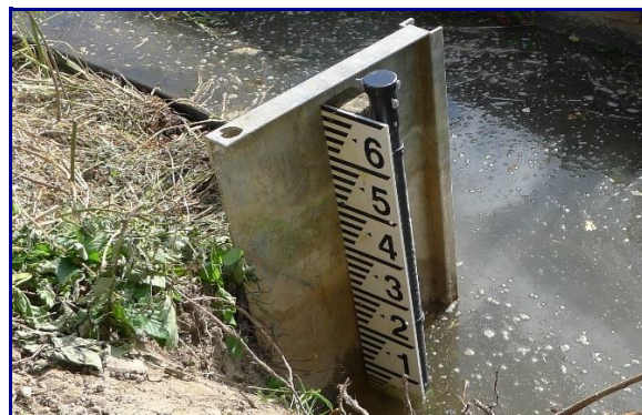
Staff Gauge and Stilling Tube on upstream wingwall, with 90 degree V-Notch plate removed
