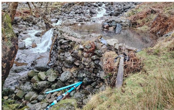
Side-channel dam and pipe offtakes in Stickle Ghyll
